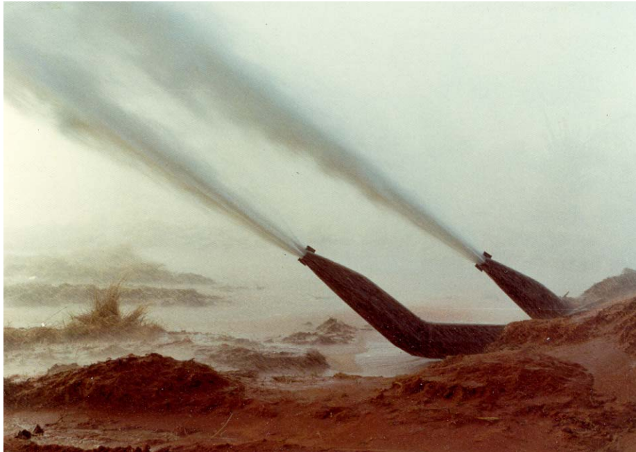
Figure 7 – Spray nozzles used for disposal of hydrostatic test water in Moomba–Sydney Binerah Downs (Courtesy of Max Kimber, 2004).
