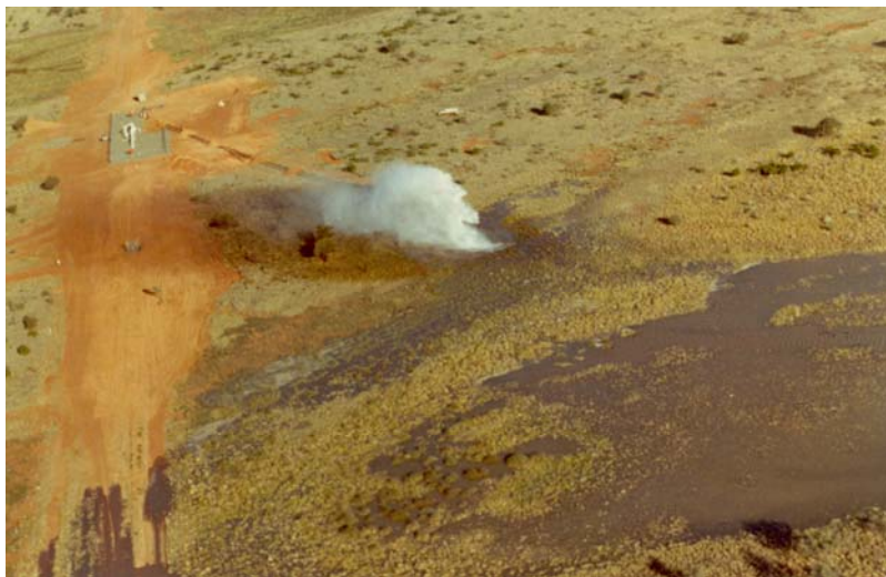
Figure 8 – Aerial view of hydrostatic test water sprayed in Moomba–Sydney Binerah Downs (Courtesy of Max Kimber, 2004).
